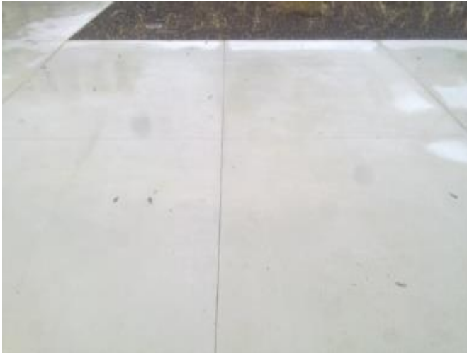
Too slippery trowel finished surface
