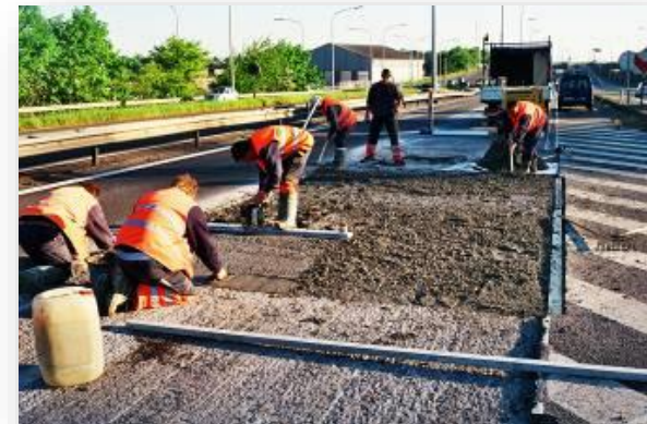
Manual pouring: too dry concrete – limited compaction
