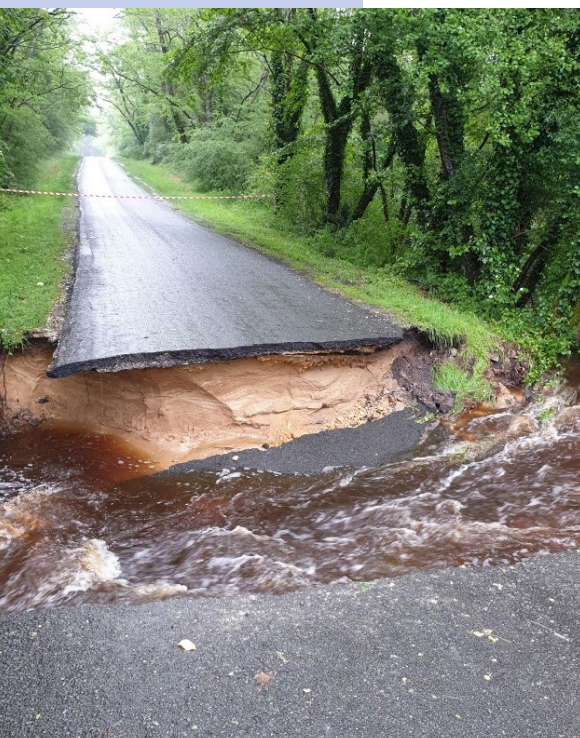
Road damaged after flooding, Gironde (France) © Facebook page of Noaillan
