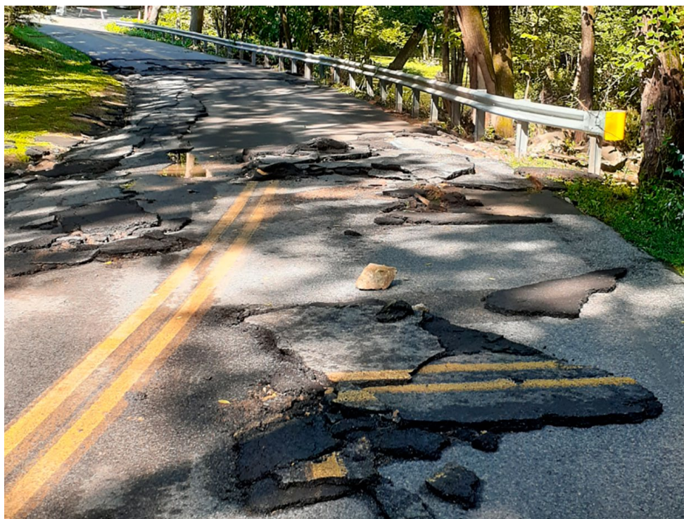
Road damaged after floodwaters, Reading Drive, PA (USA) © Rich Hawk / sauconsource.com
