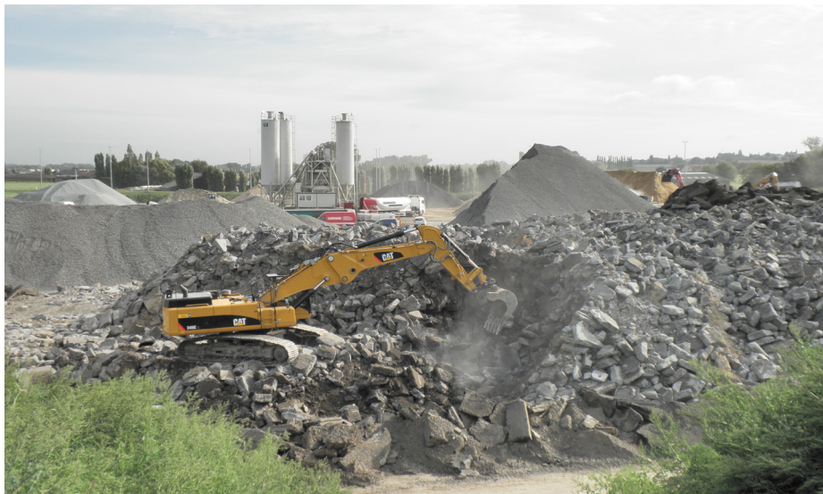
Image. Concrete demolished to be used in road base applications or in the production of new concrete for pavements.
