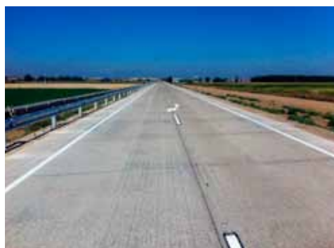
Detail of the micro-milled surface and view of the motorway in Leon, Spain Photos: IECA
