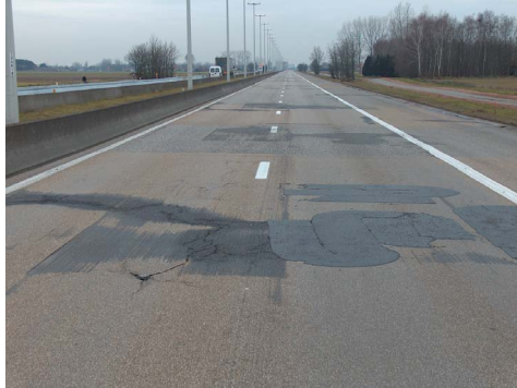
Highway in bad condition
