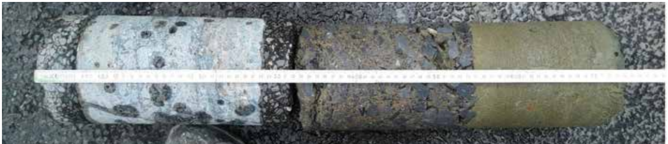
Figure 5: View on a core taken from the E40, Belgium, near Heverlee in September 2020 after almost 50 years in service. A limited degradation of the lean concrete and the asphalt interlayer is visible.
