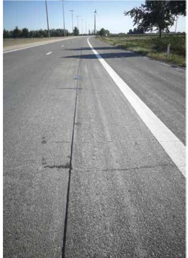
Figure 1: Regular crack pattern with the application of the saw cut as crack initiation (E34 – Kaprijke)
